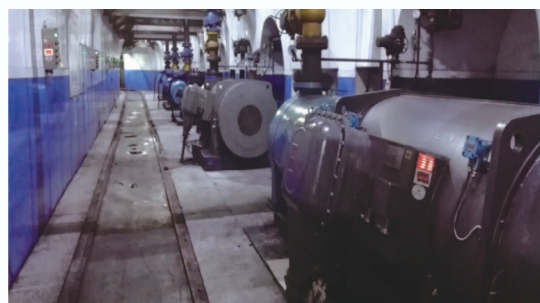
Water pump automation control system in the central pump room
